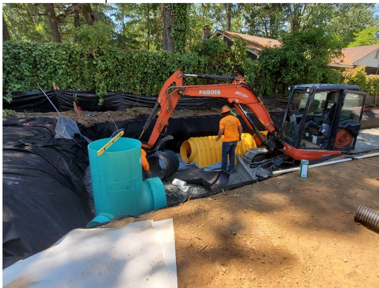
Installing stormwater system components in the trench on the west side of the library.
