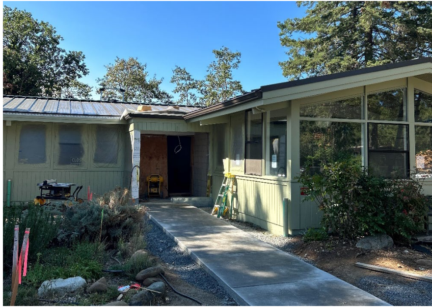
Library entrance with new sidewalk, framed vestibule, exterior paint, and metal roof.
